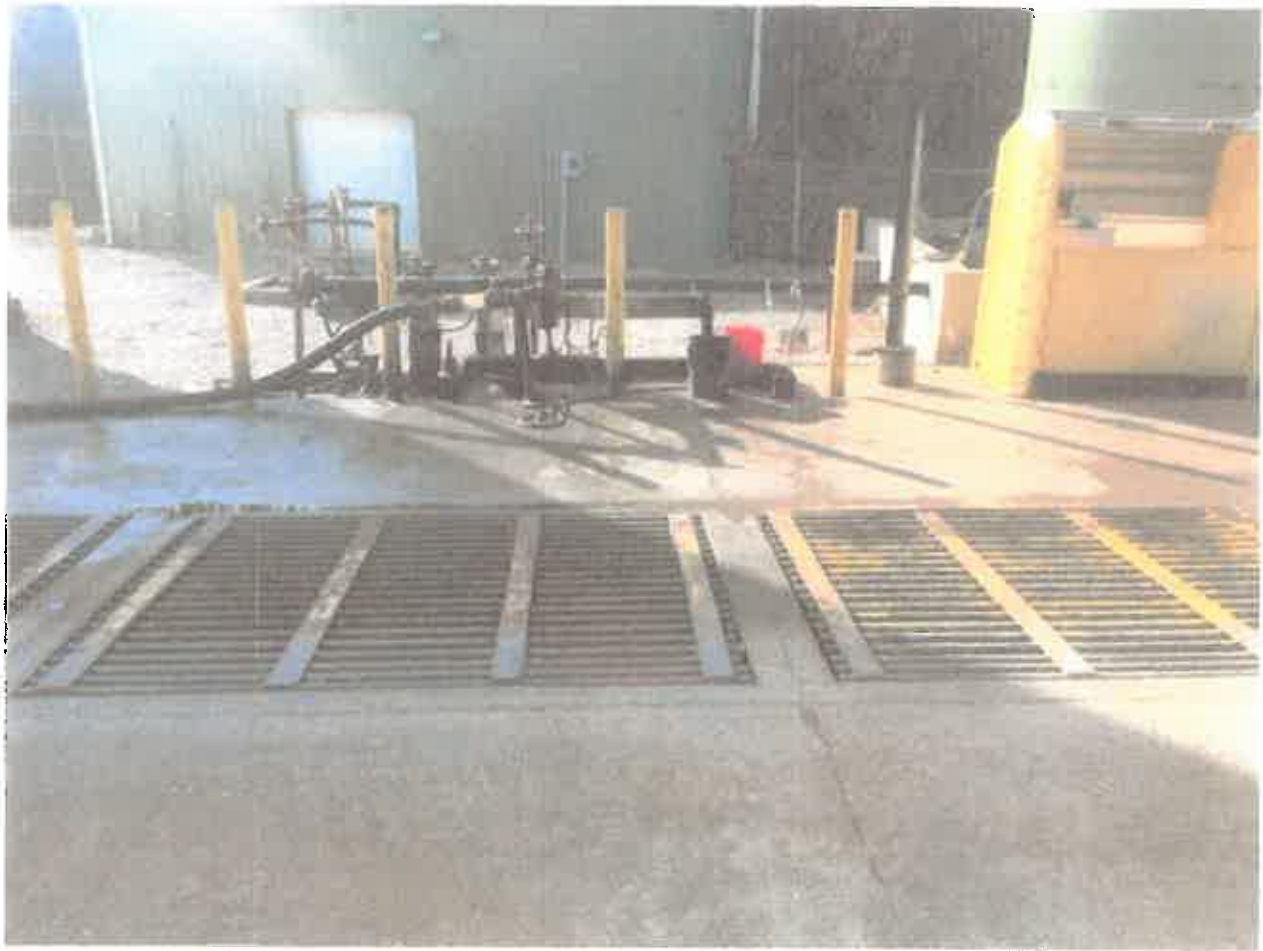
Figure 4 – Unloading pad and filtering system at the facility.
