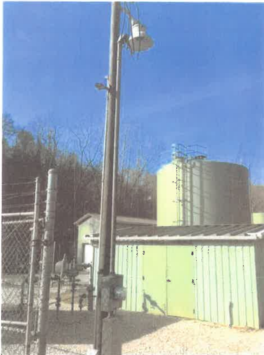
Figure 8 – Security camera on pole.
