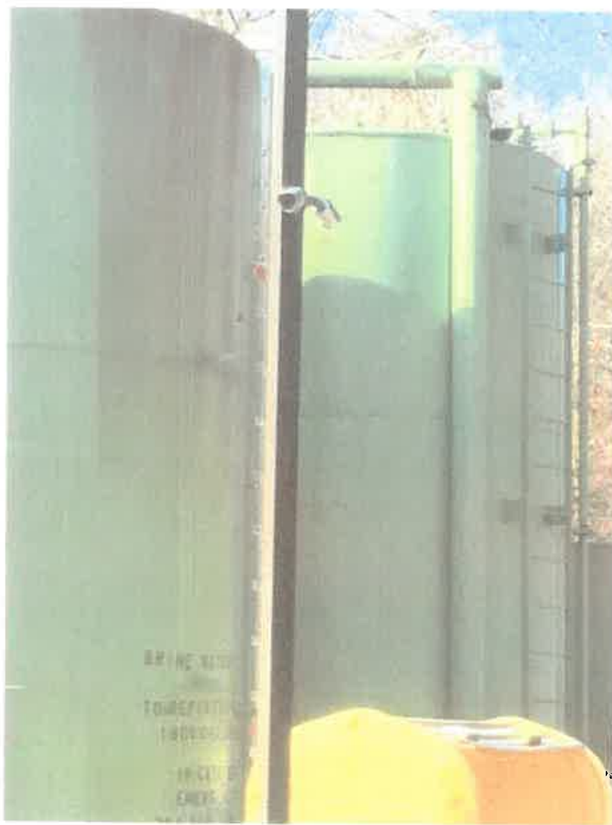
Figure 10 -- Two security cameras on pole at tank battery.
